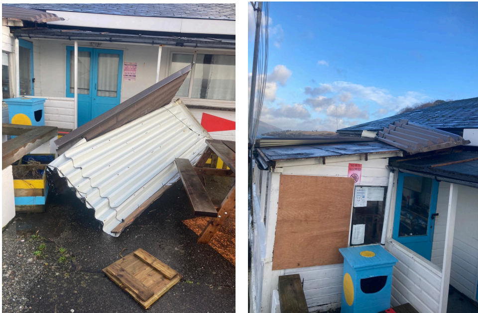
Roofing panels and window damage to bridge this month. Work party list growing
